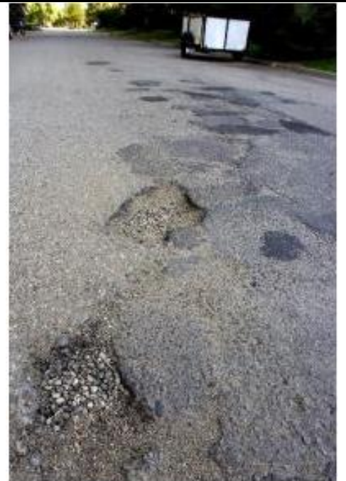
Paseo Del Prado Street in Boulder County has broken pavement and numerous road patches. ( PAUL AIKEN)
